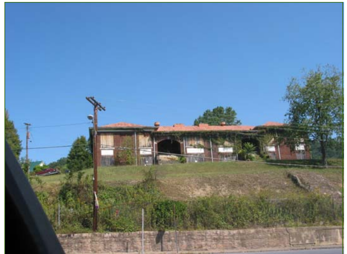
View of vacant Ansted High School Building. Redevelopment plans by the Town of Ansted include town offices, community center, and a small business center complex
