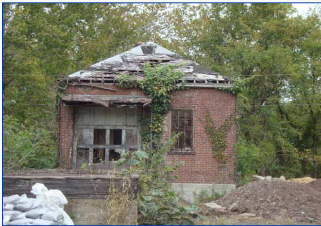
Exterior View of Former Rail Depot Building in 2008, prior to the Start of Building Rehabilitation Activities
